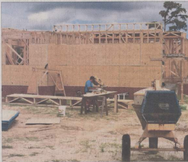
Work continues on a new house being constructed at the Riversound Development by Drummonds Point.
